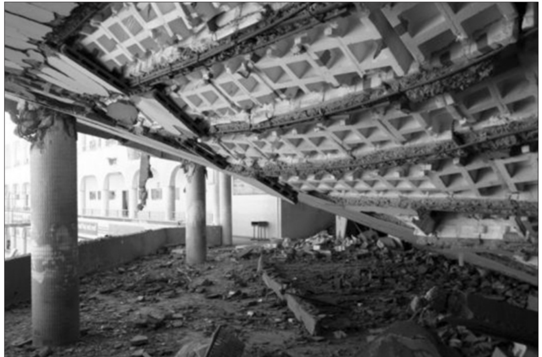
The collapsed ceiling of the Al-Arqam elementary school in Gaza City. An Israeli military spokesperson told The New Standard the school was bombed because "it was bringing up the next generation of Hamas members." © Jon Elmer 2005
